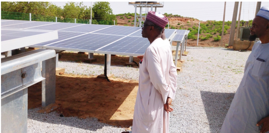
Fig 16: Prof. E.J. Bala inspecting the 60KW solar PV grid interconnected mini-grid project in Torankawa, Sokoto State by FM Power
